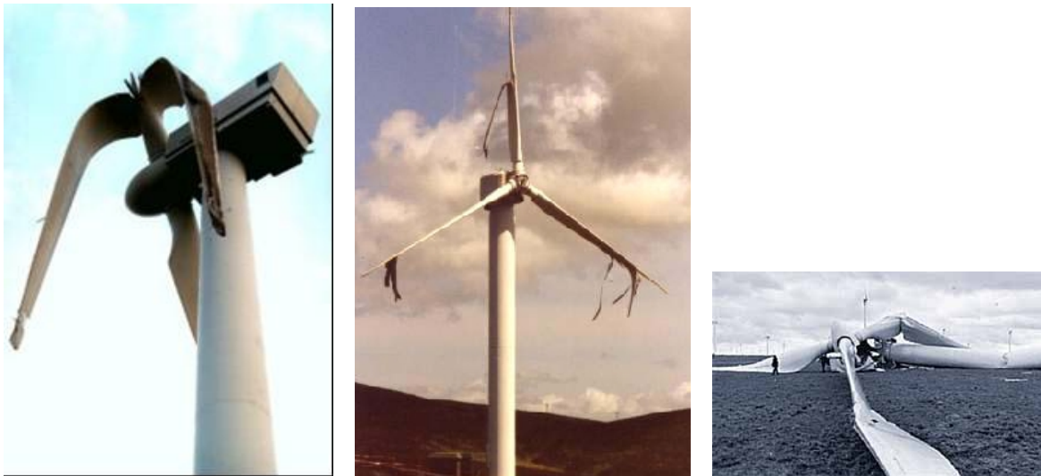
Figure 1: Examples of rare structural failures of horizontal axis wind turbines.
