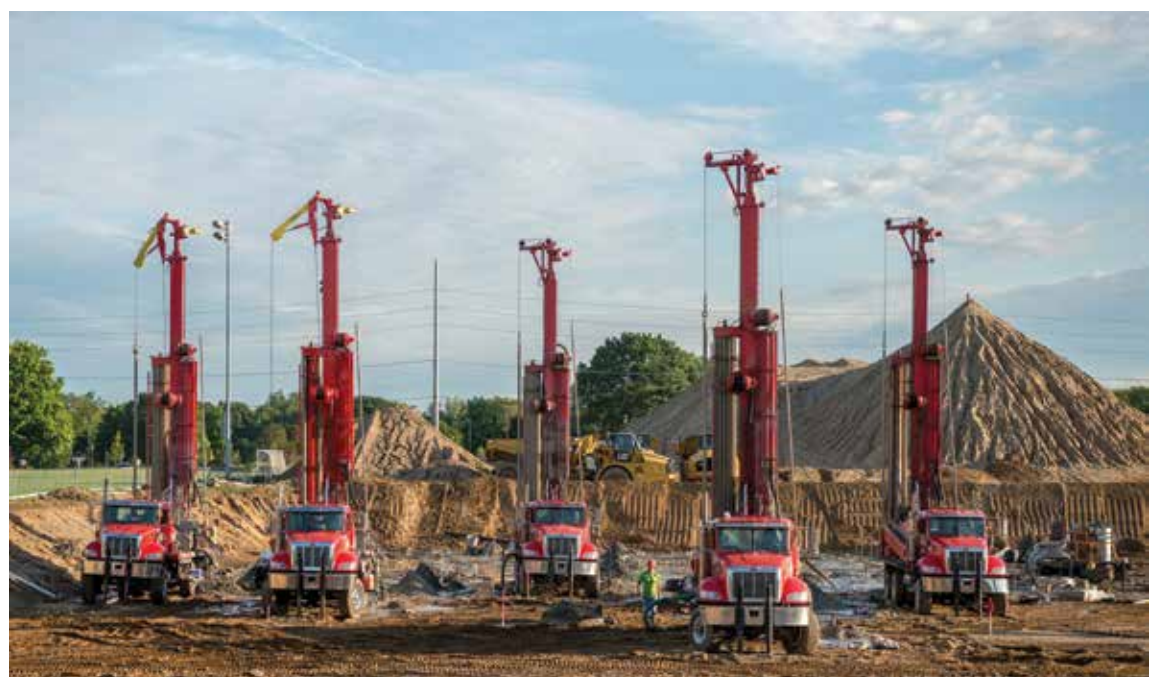
The third phase of the project, currently under construction, is the installation of approximately 650 wells and 1,350 tons of capacity under what will become the new Ricci Athletic Fields on the north end of campus. This system will connect to a new remote chiller plant to be located just east of Wilson Drive.
