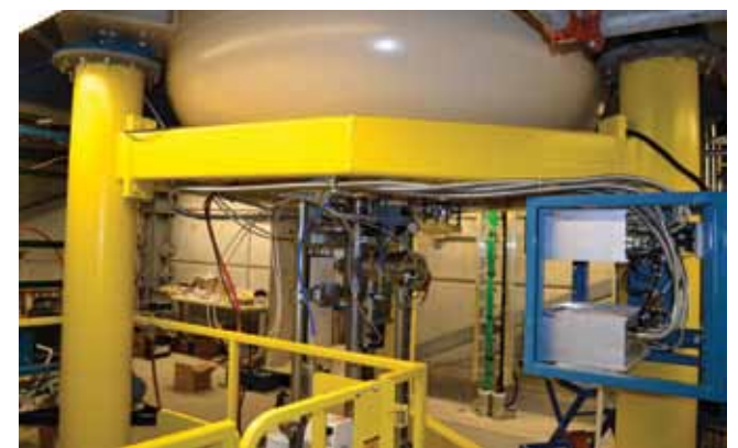
The accelerator tank, in position in the basement of Nieuwland. The tank itself is about 21 feet tall, but the tower rises approximately 40 feet above the existing roof of Nieuwland Science Hall.
