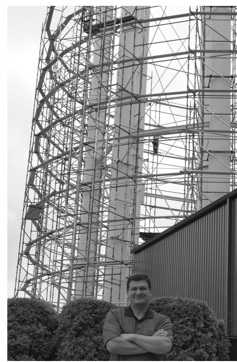
Utilities director Paul Kempf stands at the physical beginning of a long stretch of summer projects. Scaffolding being mounted around the water tower will support protective covering as it is stripped and repainted beige. South of the water tower, North Quad is surrounded by fencing as new storm sewers are installed. ND Works staff photographer.
