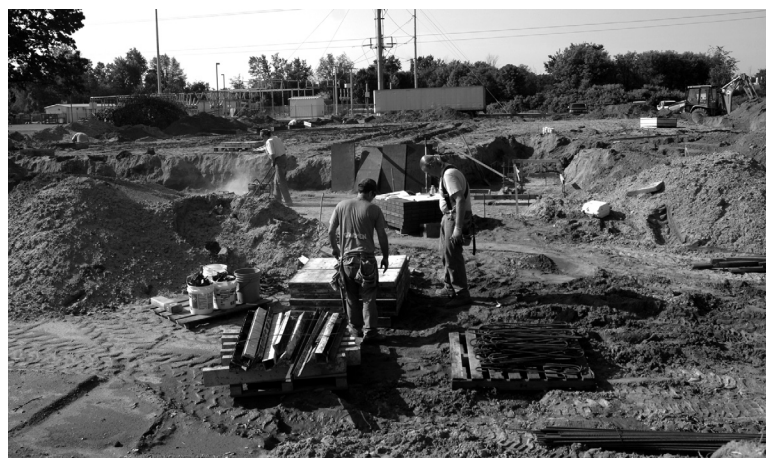
Construction on this new engineering facility at White Field is expected to be completed by fall. Photo by Joe Raymond.
