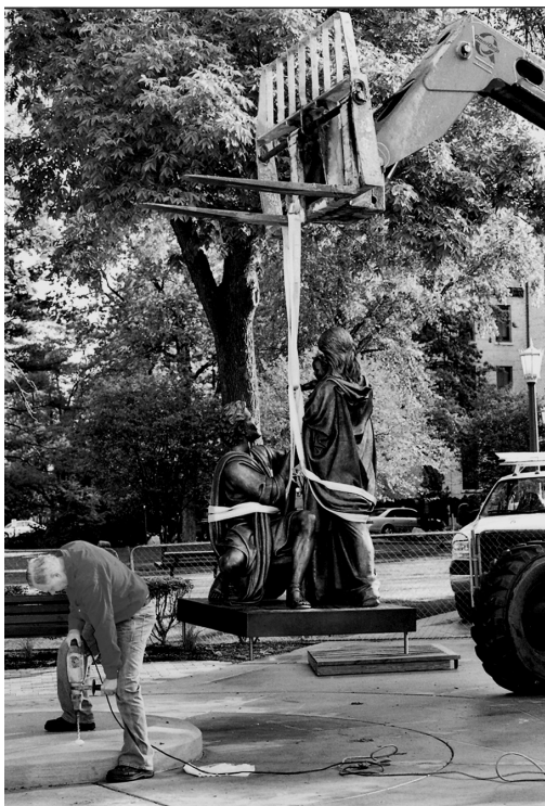
The massive sculpture was lifted into position with a crane operated by a crew from Ziolkowski Construction, South Bend. The installation was completed in a little over an hour.
