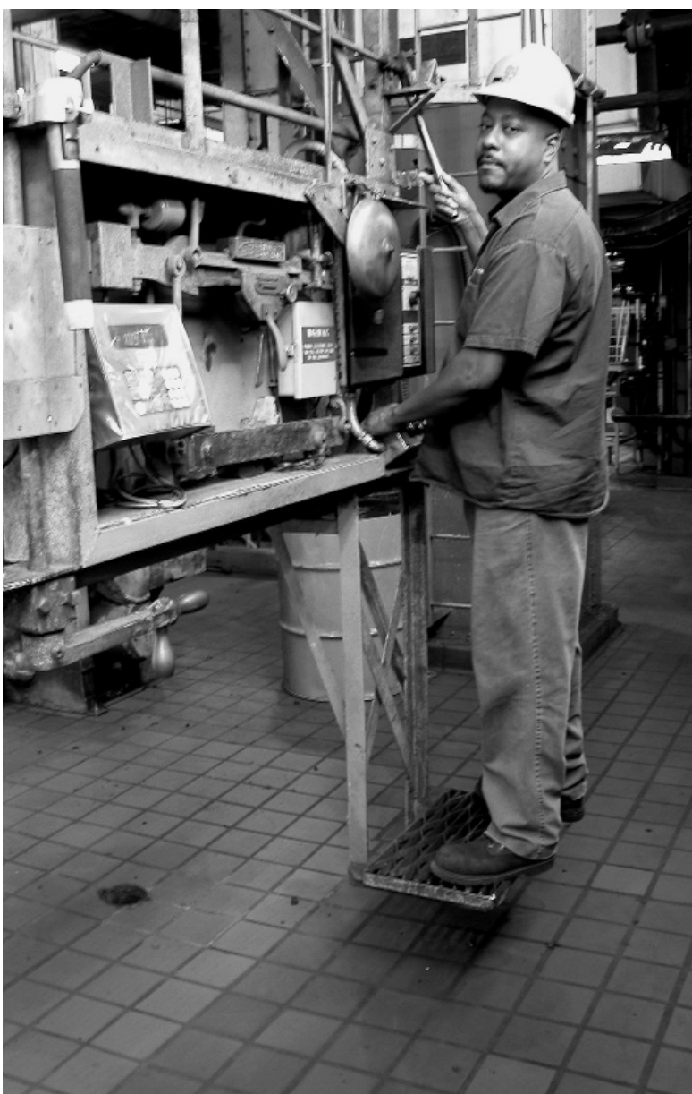
Fred Riley Jr., a boiler operator in the utilities department, slides on a coal lorry while lifting levers that deliver coal to the boiler. The boiler produces steam, which in turn drives a compressor that produces chilled water. The chilled water is then pumped to campus buildings for air conditioning. ND Works staff photo.
