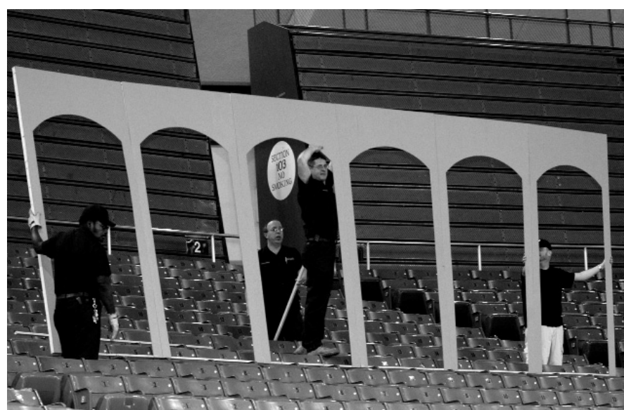
A building crew puts the first touches on a backdrop meant to harken the bullfighting rings of Spain. Photo by Rebecca Varga.
