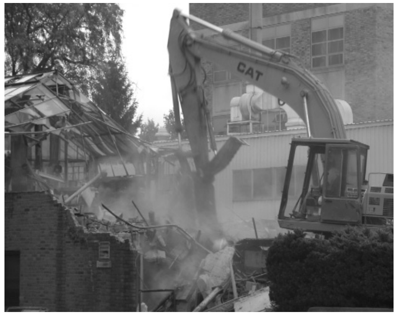
The old biology greenhouse, pictured at the far left as it looked for 50 years, comes down, above, during two days of demolition late last month. ND Works photos
