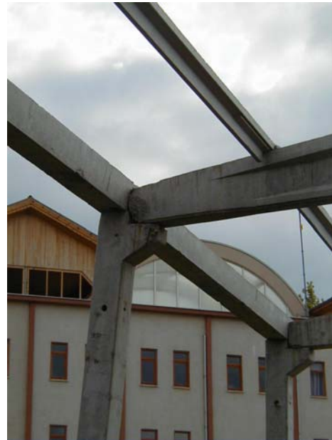
Figure 4 Impact damage near the roof level
