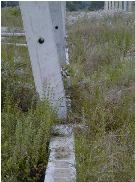
Figure 3 Flexural hinge at the base of a precast column
