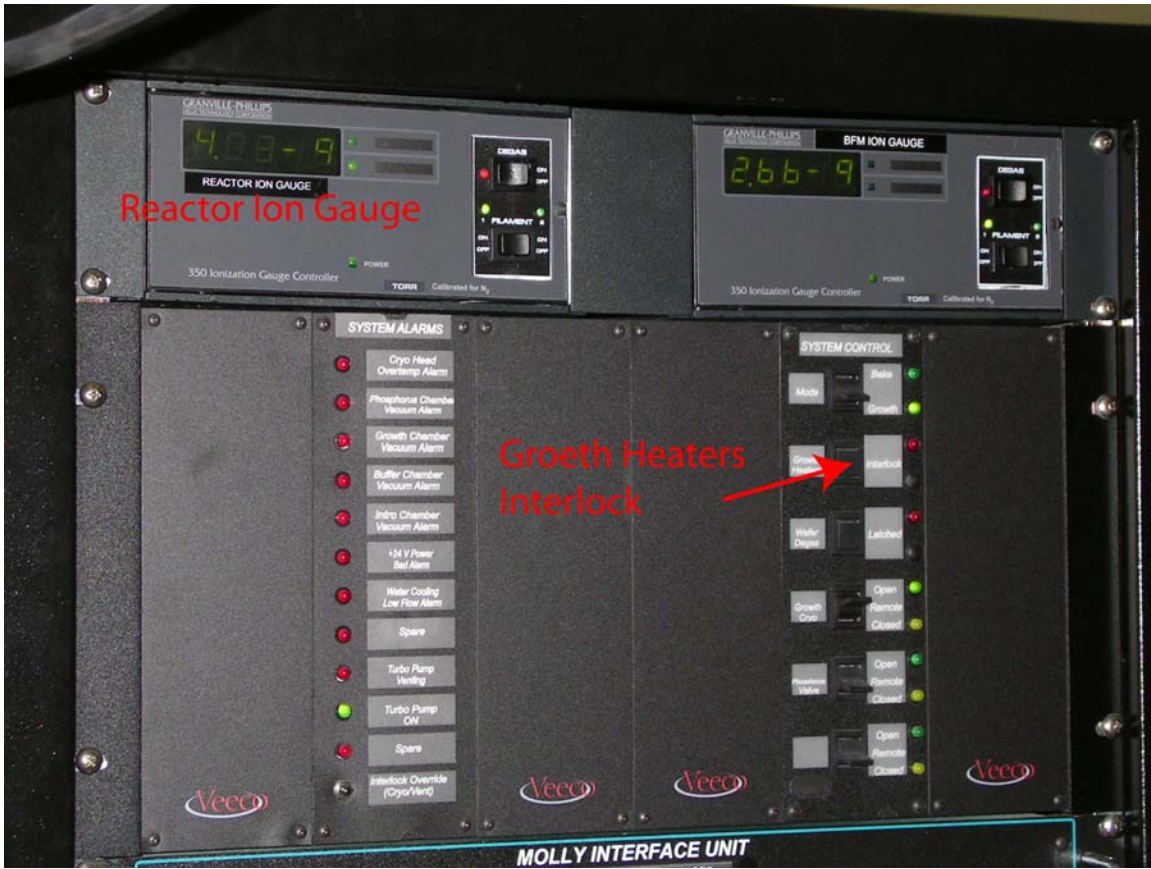
Figure 2: Reactor and Beam Flux Monitor Ion gauge (top). System alarms and interlocks (bottom left and right).
