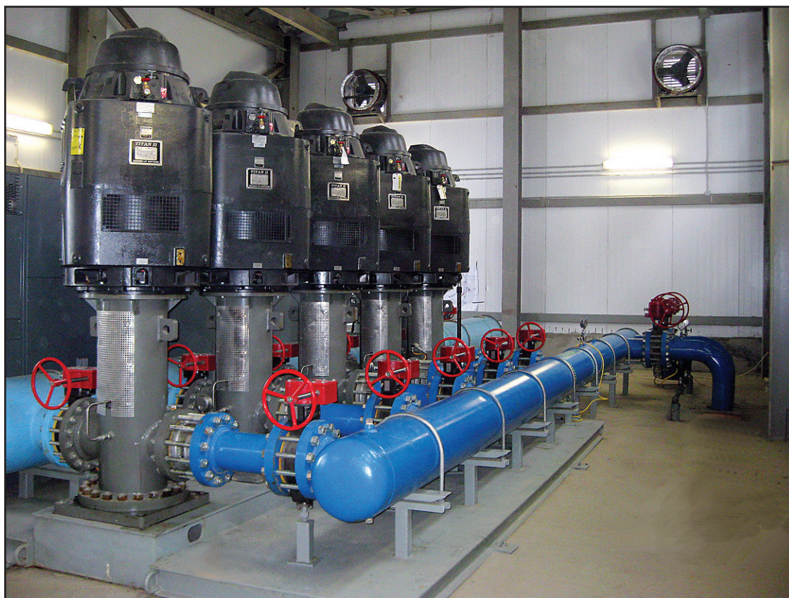
BOOSTER PUMP STATION — Torrent designed this vertical turbine booster pump station to be used at Rosa Khutor Resort in Sochi, Russia, site of the 2014 Winter Olympics. (Photo provided)
