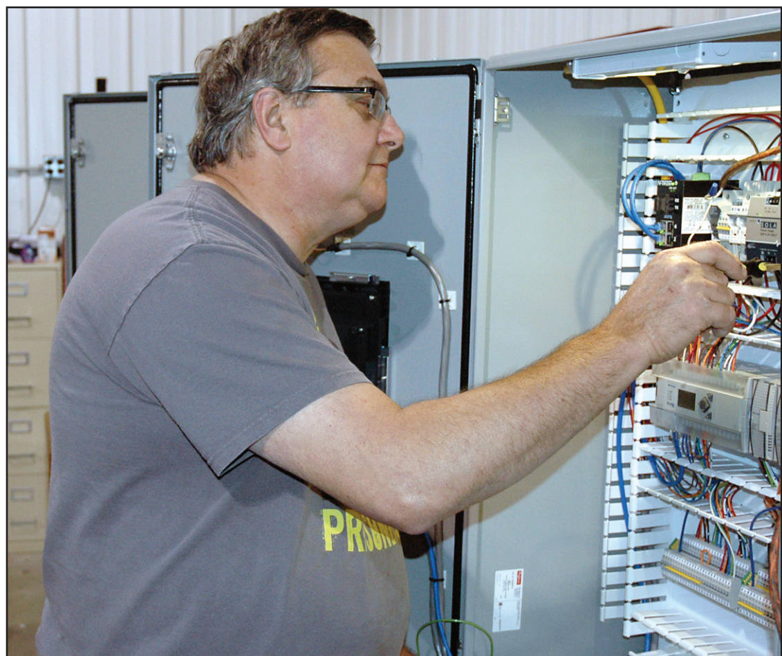
PUMP STATION BRAINS — Keith Wellbaum of Torrent Engineering and Equipment works with an industrial logic control system that will be the brains for a pump station. (Photo by Tim Ashley)
