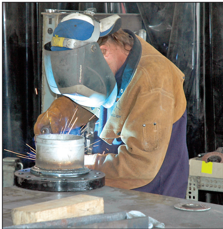
ON THE JOB — Ted Grumme welds a high pressure pipe spool for Torrent Engineering and Equipment. (Photo by Tim Ashley)
