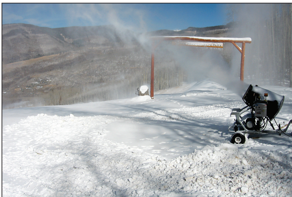
SNOW MAKER — Torrent Engineering and Equipment designed the pump station delivering water to this fan snow gun at the Golden Peak skiing race course at Vail Mountain Resort in Colorado. (Photo provided)
