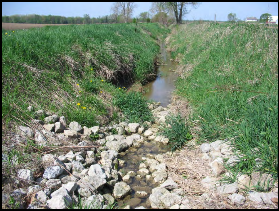
Grade control structure installed along Dillon Creek through the Watershed Land Treatment Program with the cooperation of the Noble County Surveyor's office.
