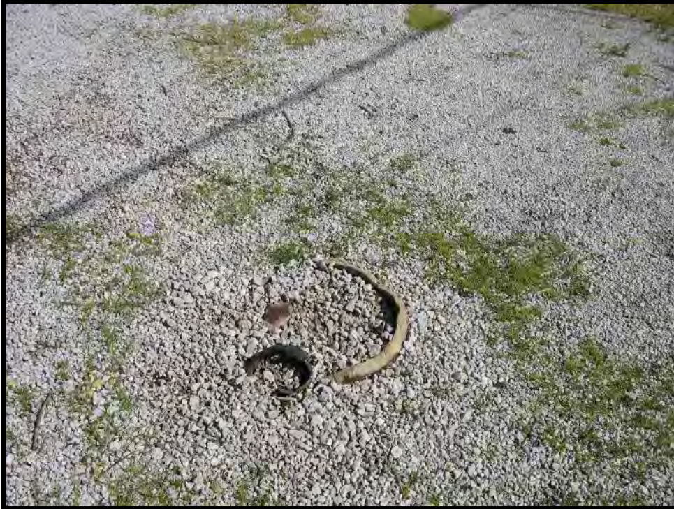
Figure 5.3. Gravel-filled storm drain.
